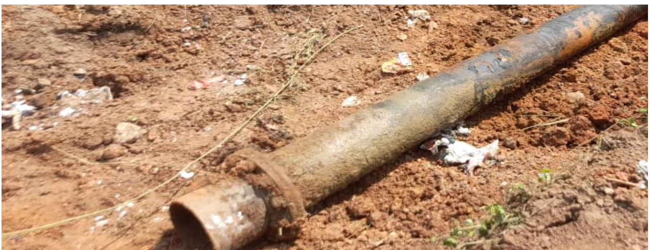
AUDC Oversight: Picture shows inadvertently excavated water pipe exposed during road construction on the Aba- Amuvi- Asaga Road
